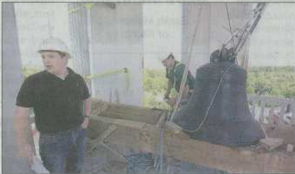
Jason Murray, left, and Matt Buckley, of Murray Brothers Construction Co., talk about the church bell, made in the early 1800s.
