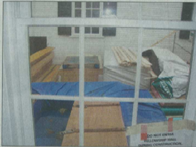
A window in Fellowship Hall shows the distance between it and the Sanctuary. Building materials lie in wait on the ground below. STAFF PHOTOS BY JOYCE PELLINO CRANE
