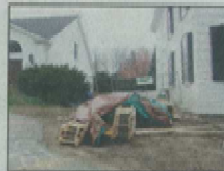
An addition is being built between Fellowship Hall and the historic Sanctuary at the First Parish Church United. The project includes an elevator to make the older building on the right handicapped accessible.
