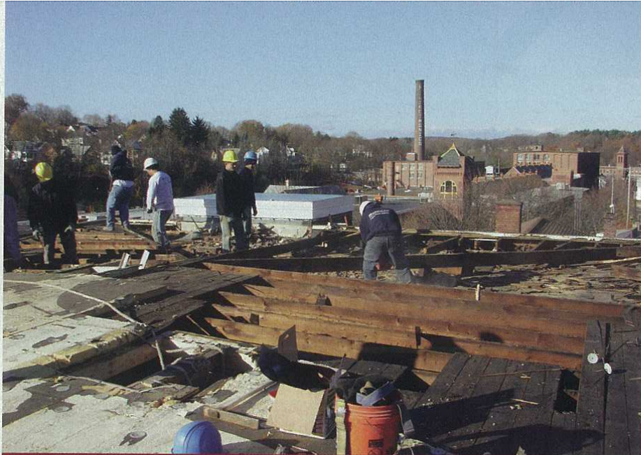
Top left: Murray Brothers Construction workers demolish roof of old mill building being converted into museum.
