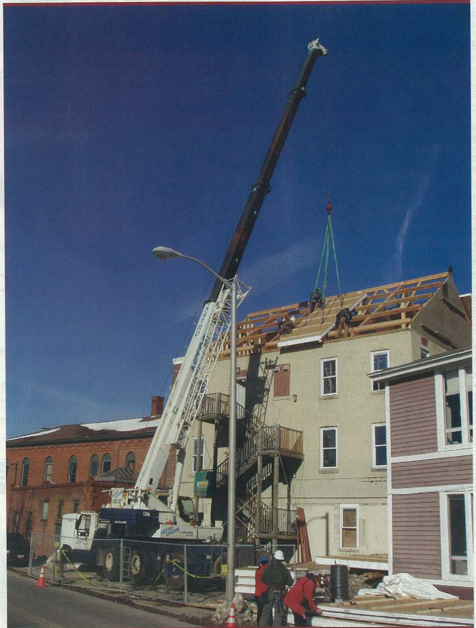
Benson Woodworking crew employs a Krupp crane provided by Astro Crane to position roof panels for Museum of Russian Icons in Clinton, Mass.
