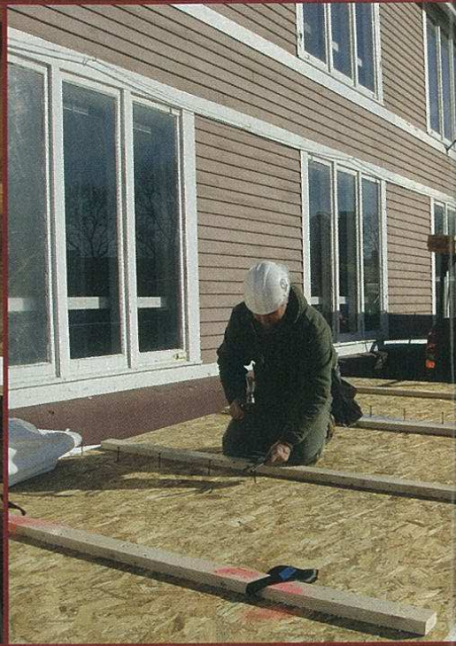
Duane Beiler pre-installs extra-long screws that will later be driven to hold panels to purlins.
