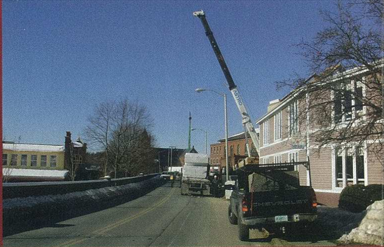
Police detail closes off one-lane of narrow section of Route 62 as crane unloads pallet of prefabricated roof panels.
